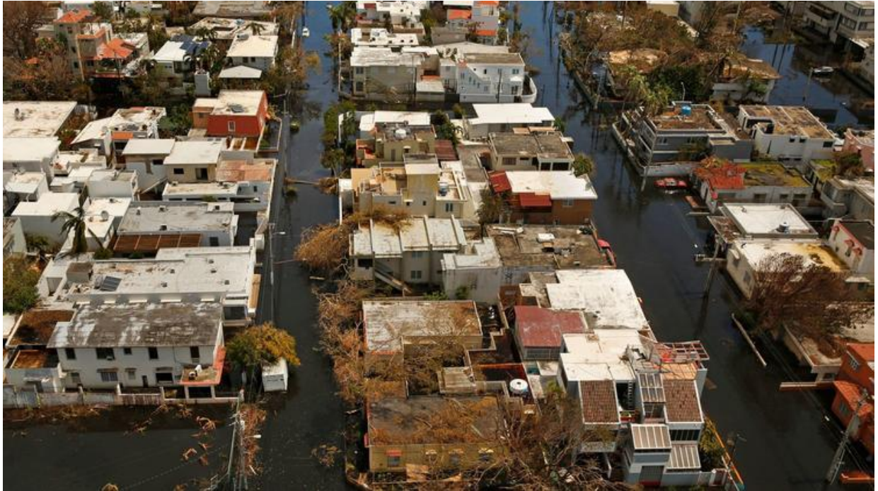
Hurricane Maria toppled electrical wires, trees and vegetation in much of San Juan, even ripping roofs off wooden homes. (Carolyn Cole / Los Angeles Times)
