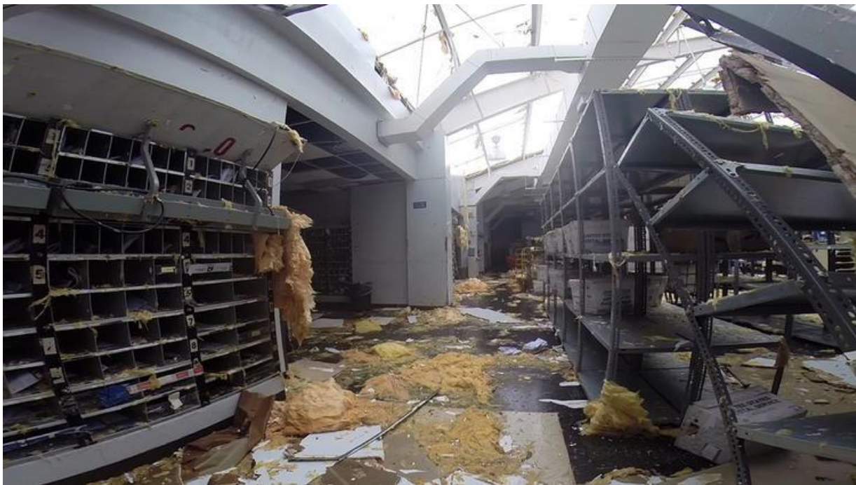
This image from video shows damage to a post office in St. Thomas, U.S. Virgin Islands. (Ian Brown / Associated Press)
