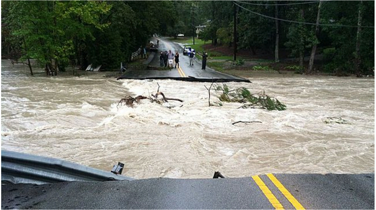
Rockbridge Road in the Columbia, S.C., area was damaged by floodwaters on Sunday. (Facebook Photo/Gills Creek Watershed Association/Erich Miarka)
