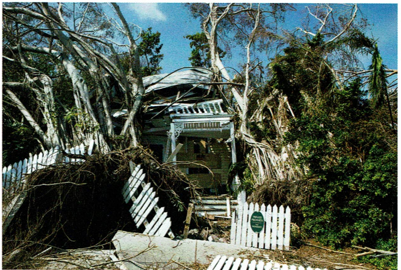
Residential property severely damaged by Hurricane Irma in Key West, Florida, on Monday, September 18, 2017.
